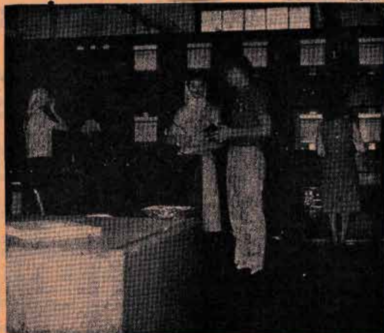
Chemistry and physics students examine the control room at the Grand Tower Electrical Station. From this central room the generators are manipulated to increase or decrease electrical output. The students above are reading some of many graphs.
